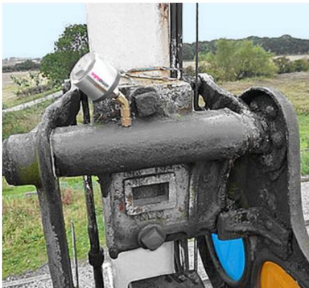
The plain bearing of a railway signal is automatically and continuously lubricated by a 30ml simalube lubricator.
