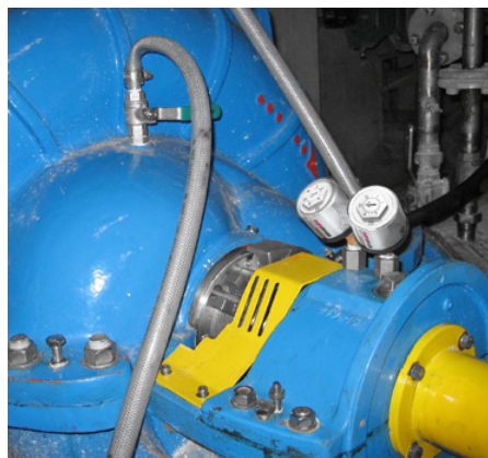
Two 30 ml simalube units lubricate the bearings of a pump.
