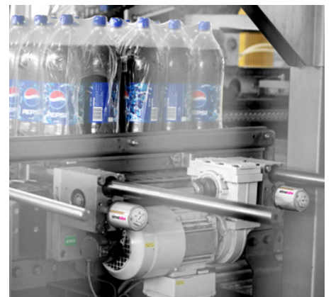
The bearing on the gear box is lubricated with two 60 ml simalube lubricators.
